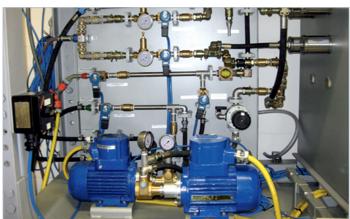
Hydraulic control systems
